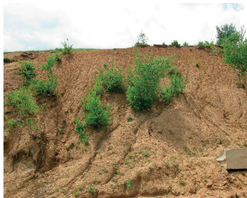
Figure 2. Surface erosion - Trickles in Novaci-Rinca area, Gorj County
